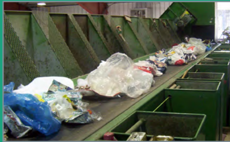
SORTING CONVEYOR BINS AND CHUTES
